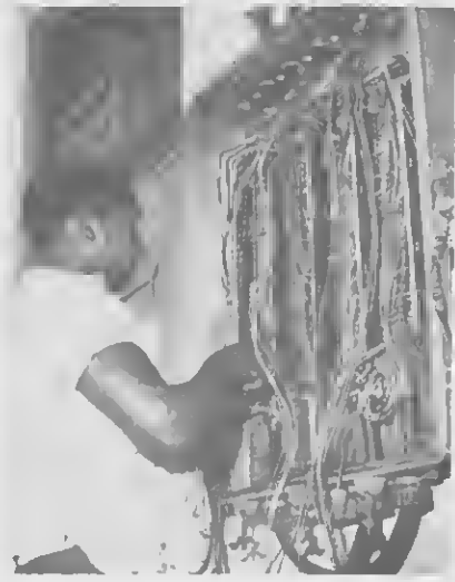
CABLES FROM crude tanks in system are tied into cables from receivers by Clinton Lynch, electrician helper A.
